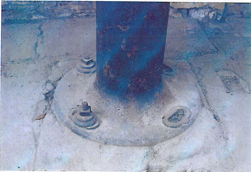
Photograph N7 – The cast-iron base of the Depot's semaphore mast was originally anchored by four \frac{3}{4} " diameter bolts. Two have been lost to corrosion. The mast must be reanchored to its massive concrete foundation.
