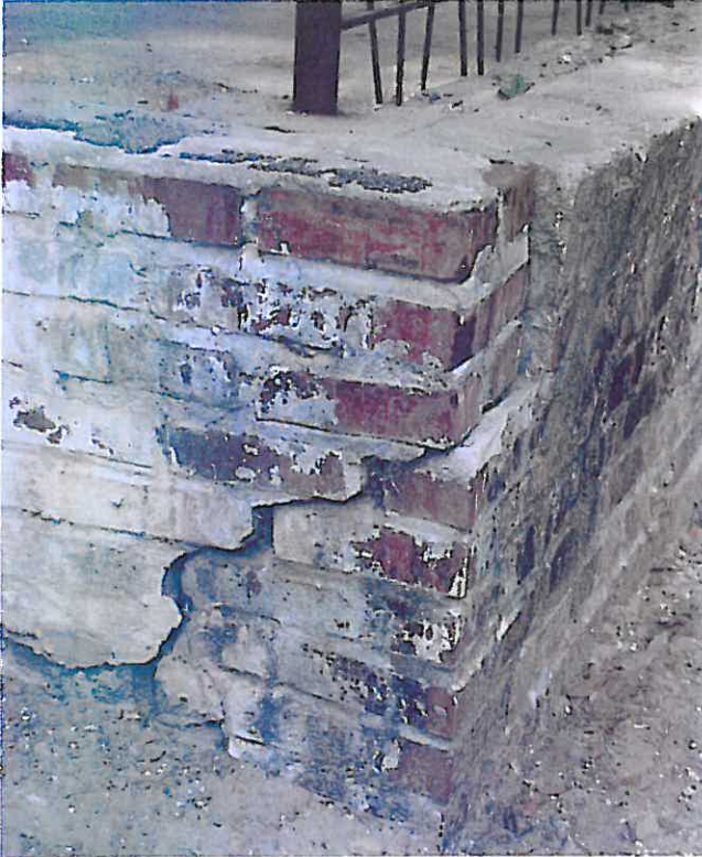
Photograph N4 – This view shows the southwest corner of the freight platform. The south wall of the platform has rotated away from the structure. A series of tie-backs will be installed to resist further movement as part of the platform deck replacement work.
