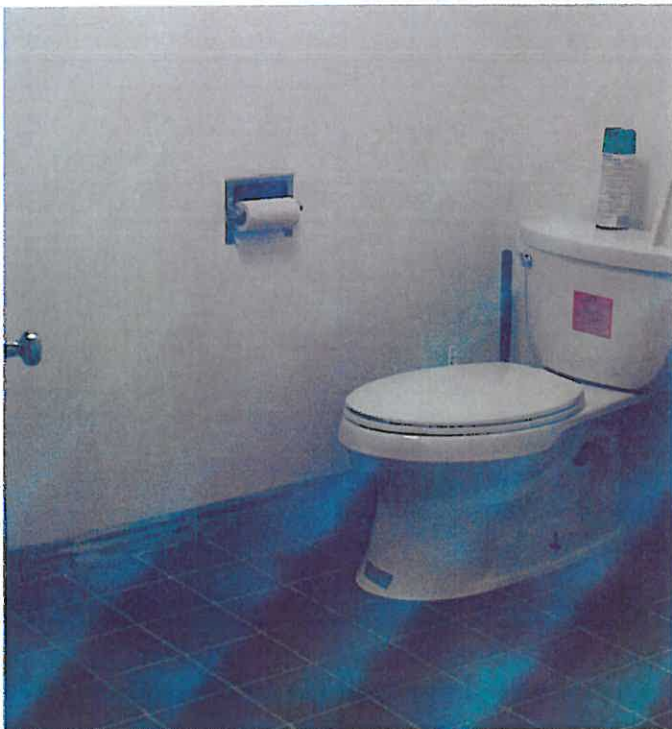
Photograph P8 – New quarry tile flooring and water closet installed in existing restroom. Further accessibility improvements will include grab rails and a new inclined mirror (already purchased and on site).
