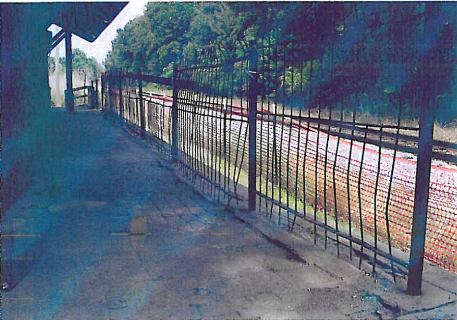
Photograph N5 – This view of the freight platform illustrates the deteriorated condition of the deck (variously mortared brick on a sand bed, concrete and asphalt). Also visible are the deteriorated platform railing, which was salvaged from a nearby cemetery in the late 1960s.
