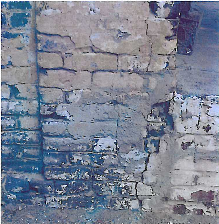
Photograph N3 – At the base of the wall, the masonry is fragmenting, no longer able to carry the load above. The existing masonry in this location will be removed to sound material.
