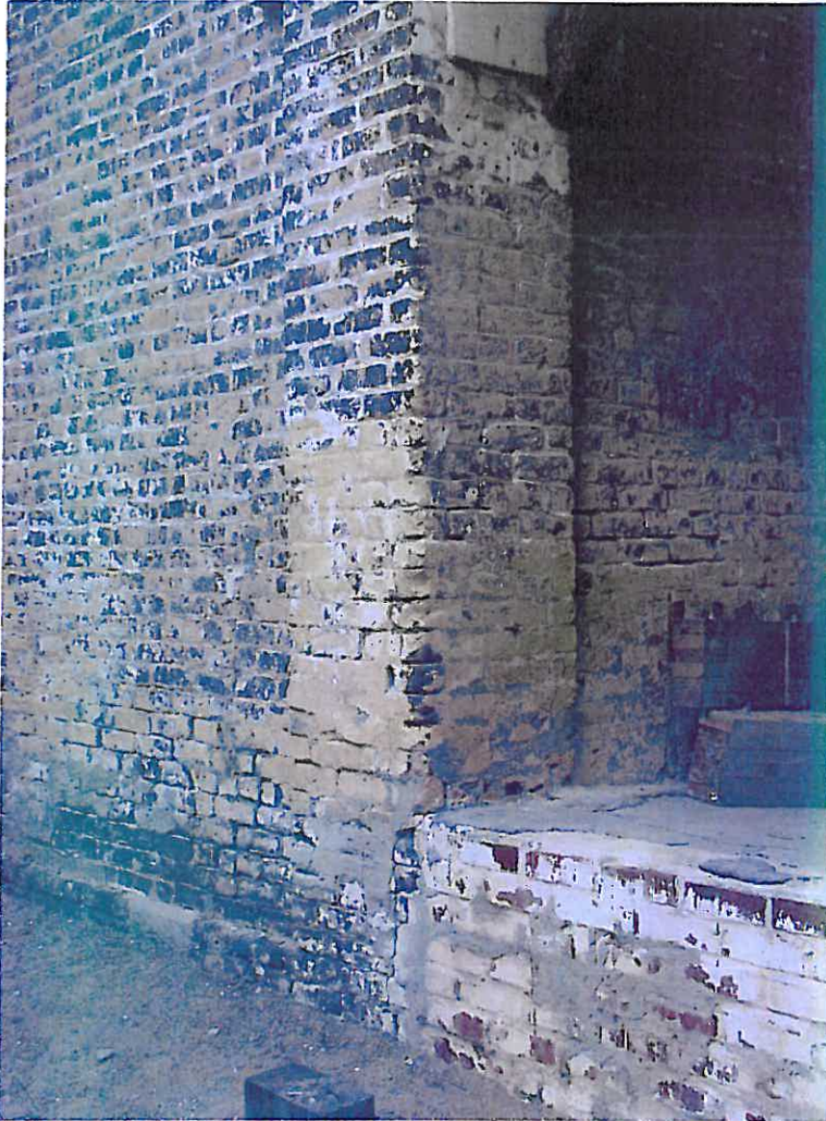
Photograph N1 – Masonry at the southwest corner of the building is failing (see the detailed images below). At this corner, the upper portion of the wall (at approximately 7' above grade) must be shored, and the large section beneath that is separating from the building and the fragmented brick at the base of the wall must be removed and replaced with matching construction.
