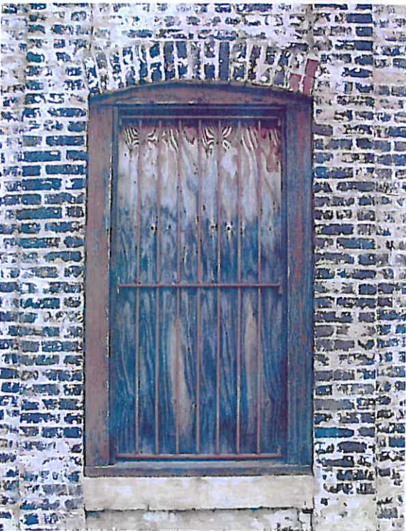
Photographs N8 and N9 – The historic wood windows require repair, reglazing and painting. In some cases, the sash are rotted and casing trim is severely deteriorated necessitating replacement. All new work will match the historic construction.
