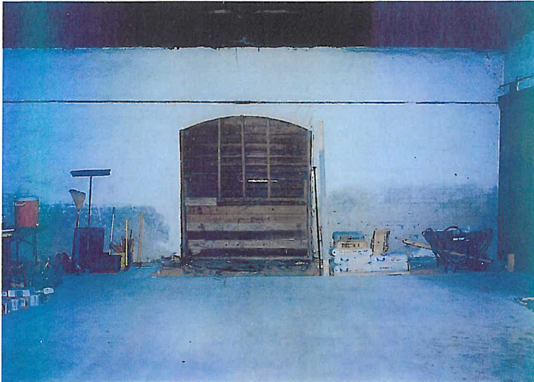
Photograph P5 -- New depressed concrete slab in Freight Room is ready for installation of new brick pavers.
