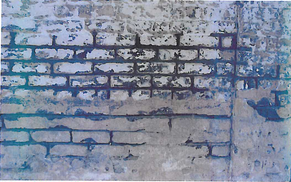
Photograph P13 – In this view, deteriorated mortar has been removed in preparation for repointing with a special low-strength mortar formulated to assure compatibility with the porous and underfired 1858 masonry units. This work is ongoing.
