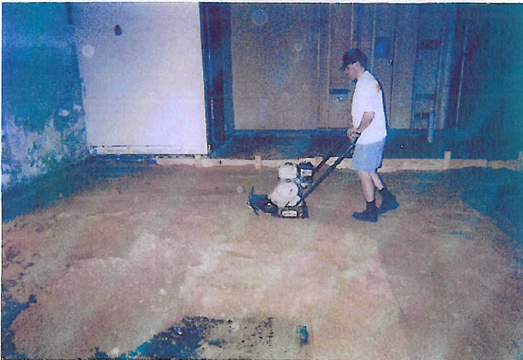
Photograph P4 – A Chapter volunteer uses a plate tamper to compact sand fill as preparation is made for placing new concrete structural slab.
