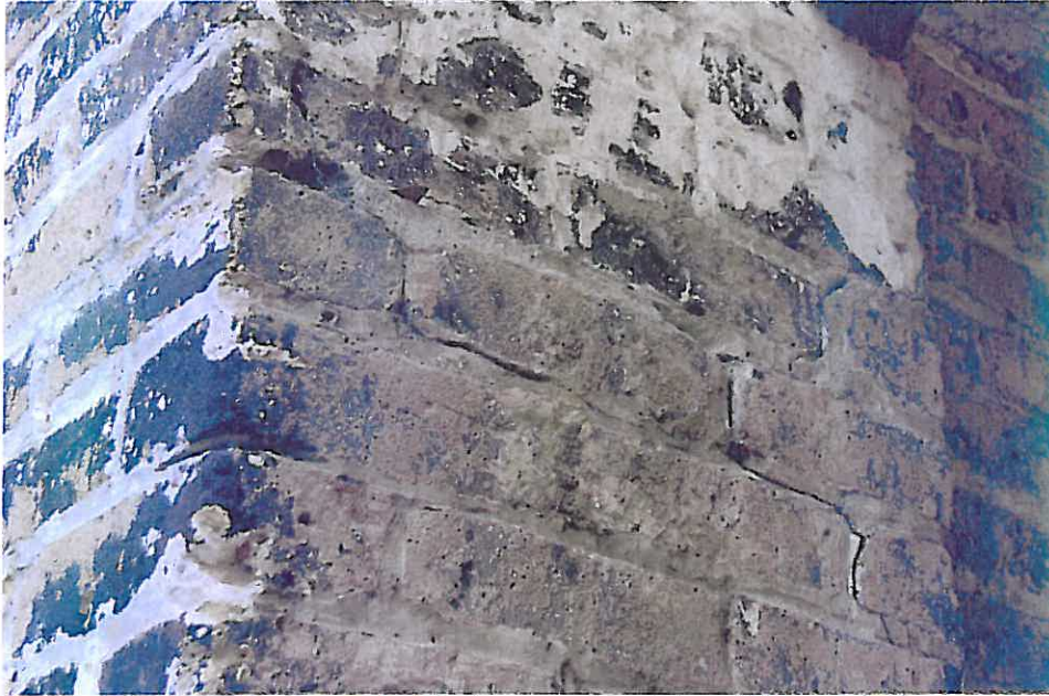
Photograph N2 – The masonry below the stepped crack has shifted outward approximately ½” in the past two years. If not addressed soon, the consequences of this progressive condition will be catastrophic. Temporary shoring will be installed by June 2011 to minimize damage in the event that the loose masonry falls. This deterioration is believed to be due in part to vibration from rail traffic.
