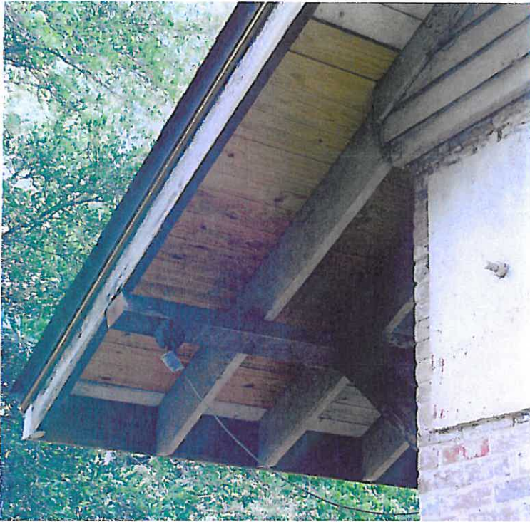
Photograph P11 – Recent roof deck repair and fascia replacement work is visible at the broad overhangs that are character-defining features of the Depot. The decking is 6" shiplap material milled by Chapter volunteers.
