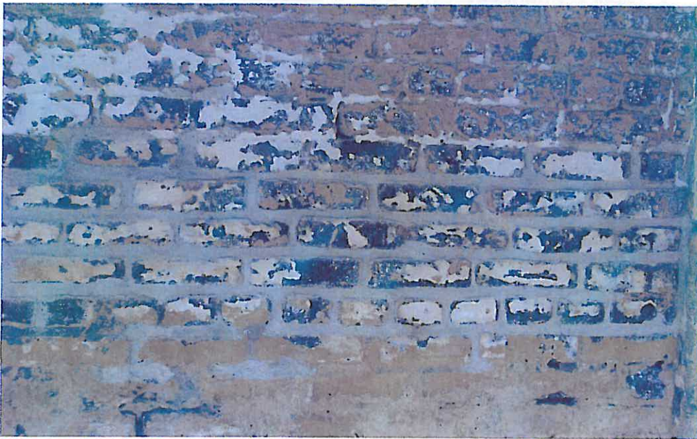
Photograph P14 – Masonry repair is being accomplished by a group of Chapter volunteers under the direction of a volunteer preservation architect. In this view, repointing has been completed on a section of the north wall.
