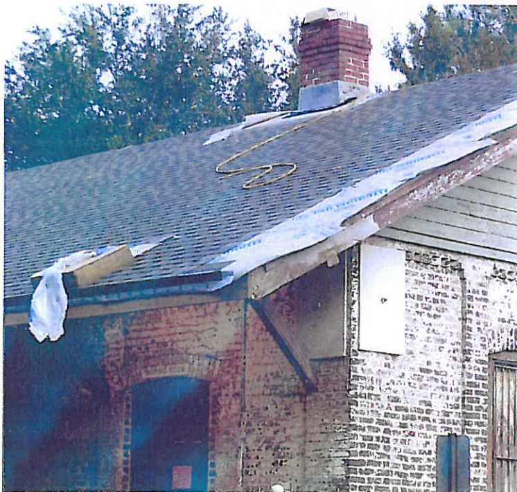
Photograph P12 – In this view, new laminated fiberglass shingles are being installed in September, 2010. The new shingles are similar in appearance to the historic wood shingles on the building prior to the 1942 fire.
