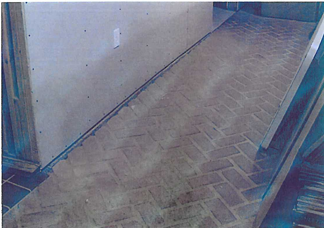
Photograph P6 -- View of completed brick floor installation in Freight Room (new restroom and office partition at left).
